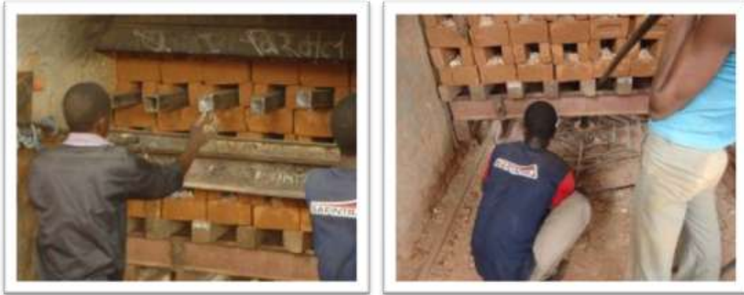
Figure 7: Lowering of unloading trolley (left); Lowering of unloading trolley on rail (right)
