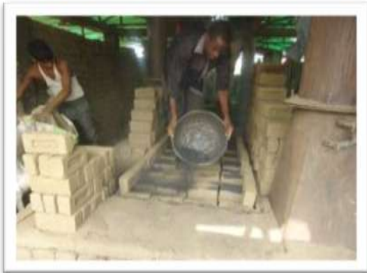
Figure 5: Coal distribution between bricks
